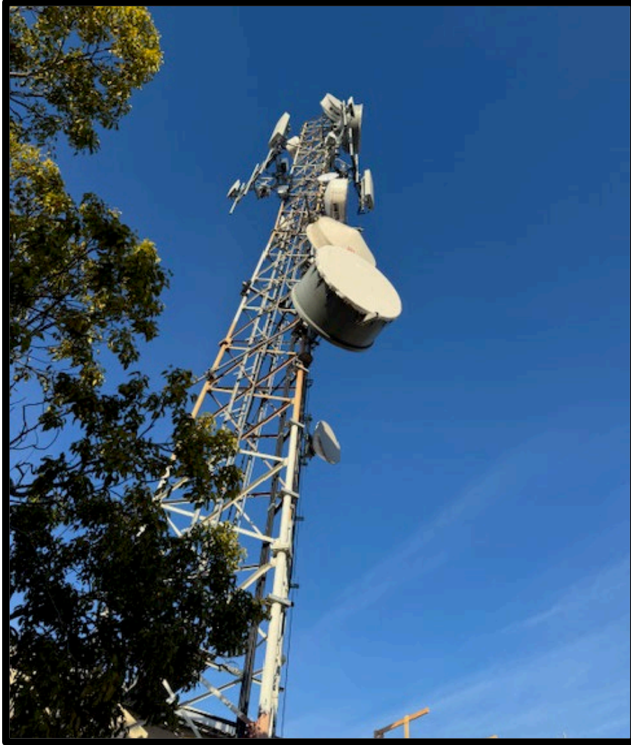
Tower in Salinas with various affixed communication Devices that are directed to the various communication towers throughout Monterey County
