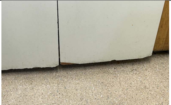
Chipped/worn out kitchen cabinetry
