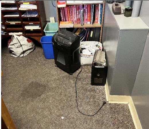
Worn out carpeting
