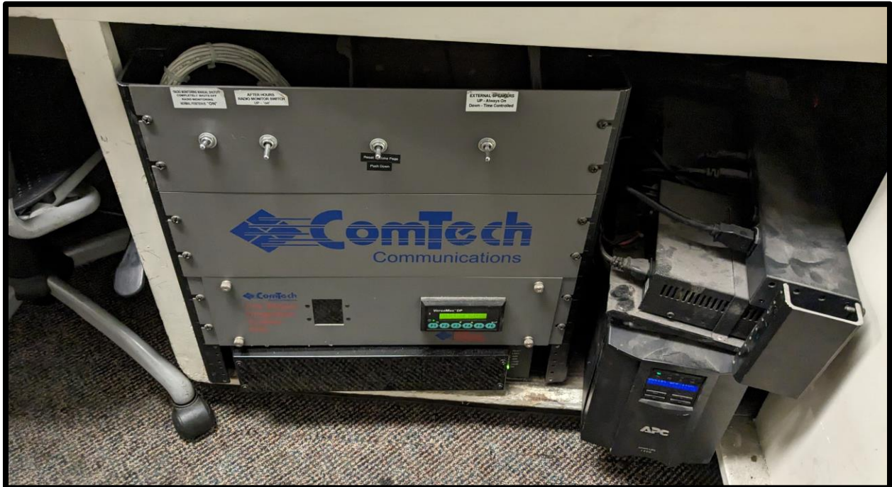
Computer Aided Dispatch alert system in Monterey Fire Station 12 Source: Photograph taken by Civil Grand Juror
