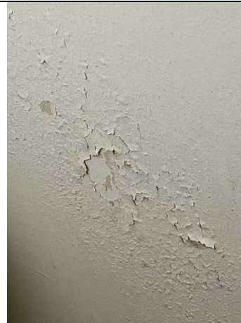
Kitchen paint flaking/peeling
