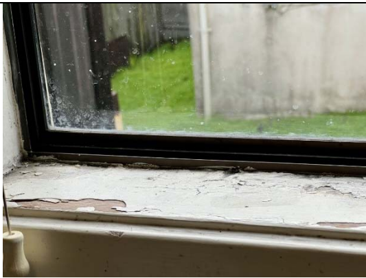
Window sill paint peeling
