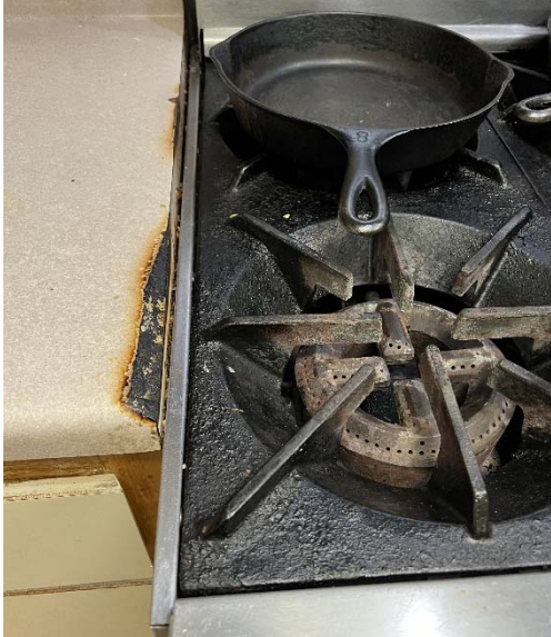
Old stove/countertop damage
