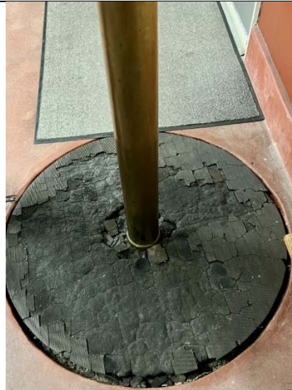
Poor condition of fire pole landing pad
