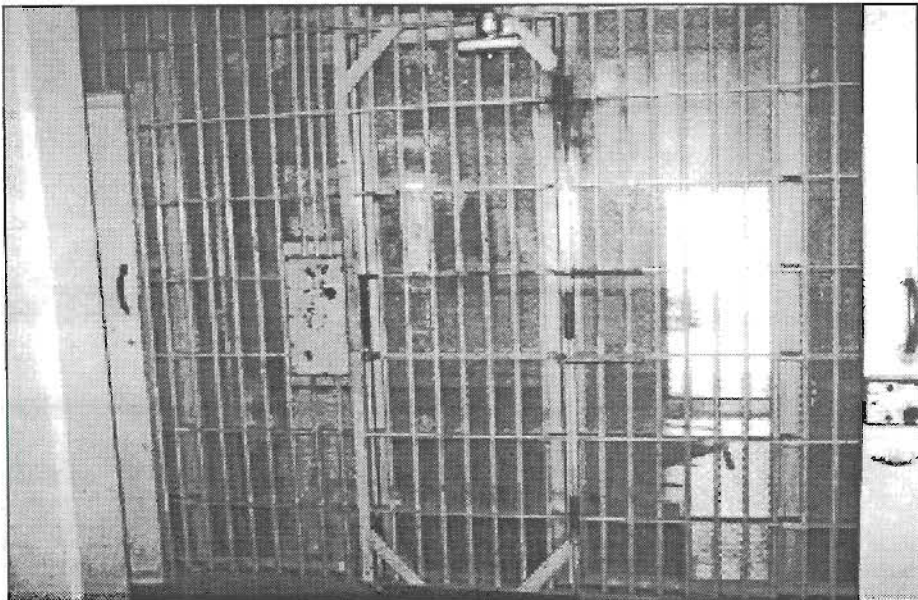
Corroded cell door.
