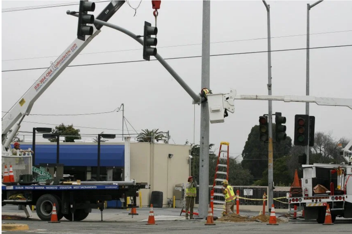
Crews work on the North Fremont Street project in 2019. (Monterey Herald file photo) Work crews install new traffic lights at North Fremont Street and Casa Verde Way in Monterey on Tuesday. (Vern Fisher – Monterey Herald)
